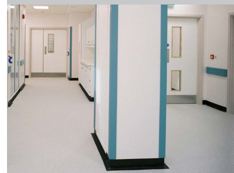
Columns within rooms and circulation areas are easily picked out by coloured edge trims.
